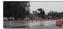
Change barriers and directional signs have been a common sight from four to six lanes (three lanes each direction). The new roadway includes a raised median, curb and gutter, and a shared-use path along the northbound lanes from Mill Road to Sherwood Road. In addition, prior to the roadway beginning, overhead utility lines were removed and placed underground along the majority of the project corridor. Perhaps the most glaring aspect of the construction work
